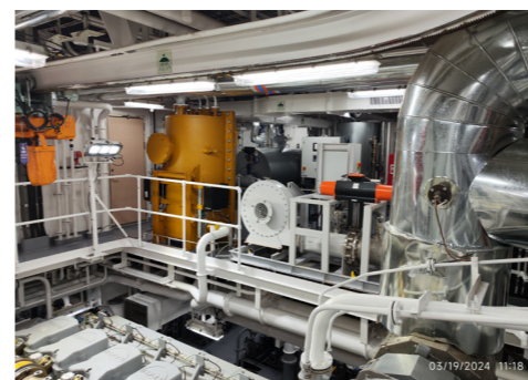
Part of main engine room
