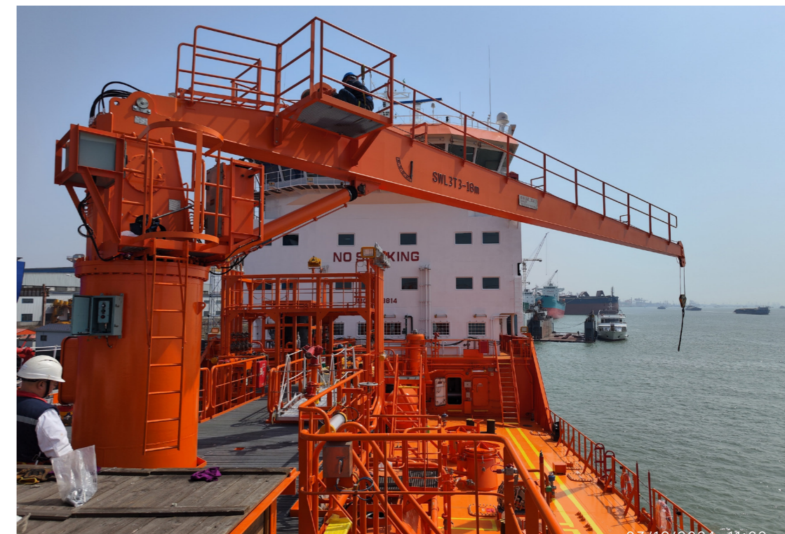
Hose crane for charging and discharging operation
